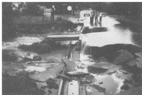
Damages to infrastructure may account for as much as 25% of the total damages incurred during flooding. Bridge damaged by flooding, Jefferson Island, Louisiana, 1979.
