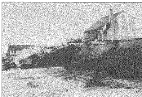
In a 1971 study, the Corps found that approximately 24% of the nation's shoreline was significantly eroding. Two-thirds of this land was privately owned. Dune erosion and house collapse, Sandwich, Massachusetts.
