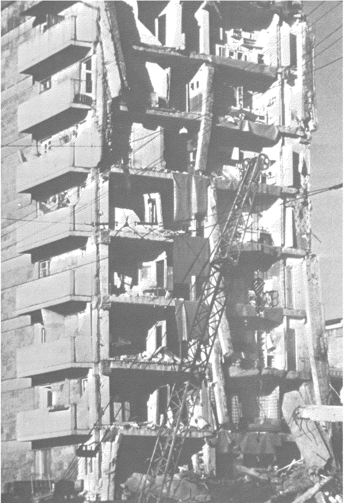
Apartment building damage in Leninakan, Armenian Earthquake, December 7, 1988.
